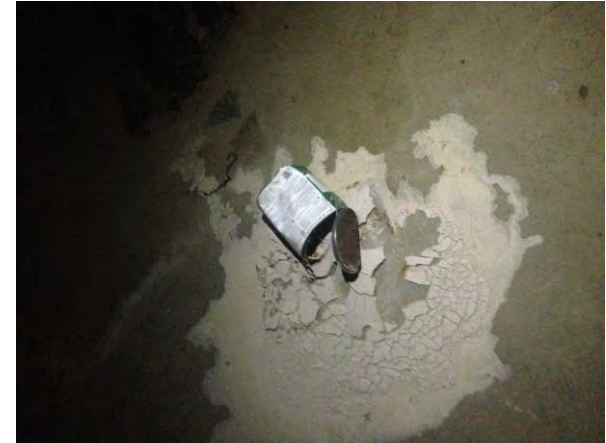
Photograph 9. View of one of multiple spilled paint containers located in the basement of the subject property building.
