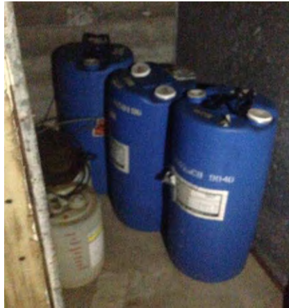
Photograph 8. View of the boiler treatment chemical containers stored in the basement of the subject property building.
