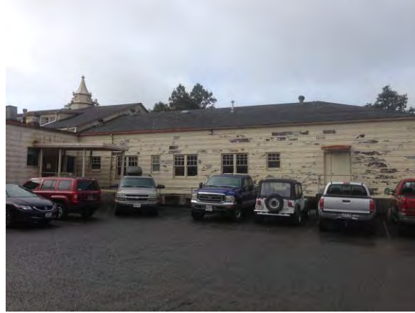
Photograph 2. View of deteriorated lead-based paint on the subject property building, from the north end of the parking lot facing west.
