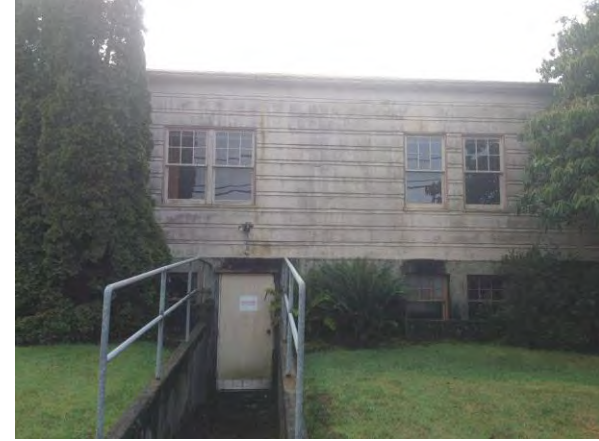
Photograph 3. View of the ramp leading to the basement of the subject property building, facing south.
