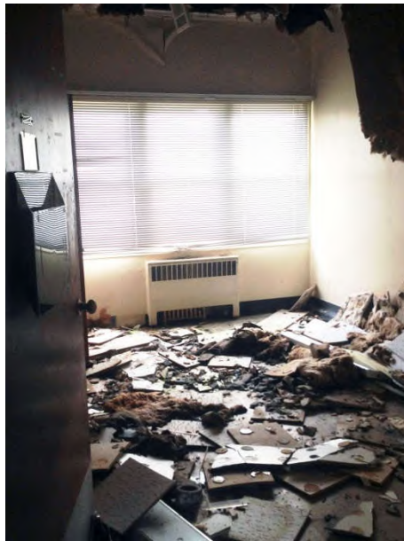
Photograph 3. A room in the main block of the Trinity Annex with collapsed ceilings
