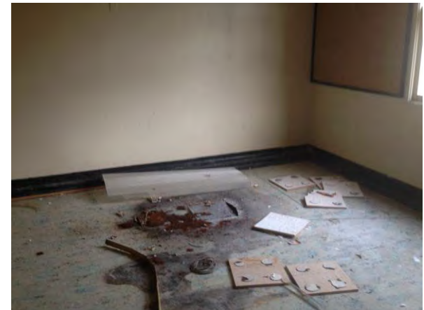
Photograph 12. View of the inside of one of the rooms with a caved-in ceiling.
