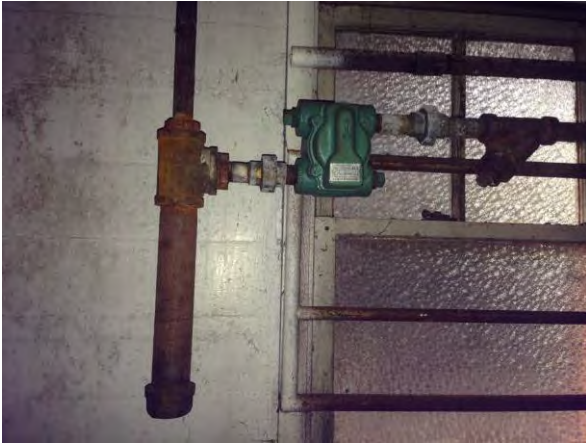
Photograph 7. View of rusted and corroded pipes in the basement of the subject property building.
