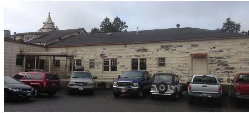
Photograph 2. View of the northern parking lot, facing west, illustrating the deteriorating condition of the building and flaking paint
