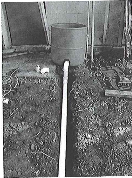
Figure 6 PVC runs from settling tank into marsh
